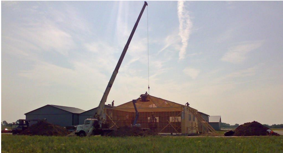
A hangar under construction using a crane, mobile lift, heavy trucks and piles of gravel and fill.
